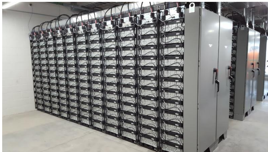
Figure 4 - Example of a BESS Enclosure 3
