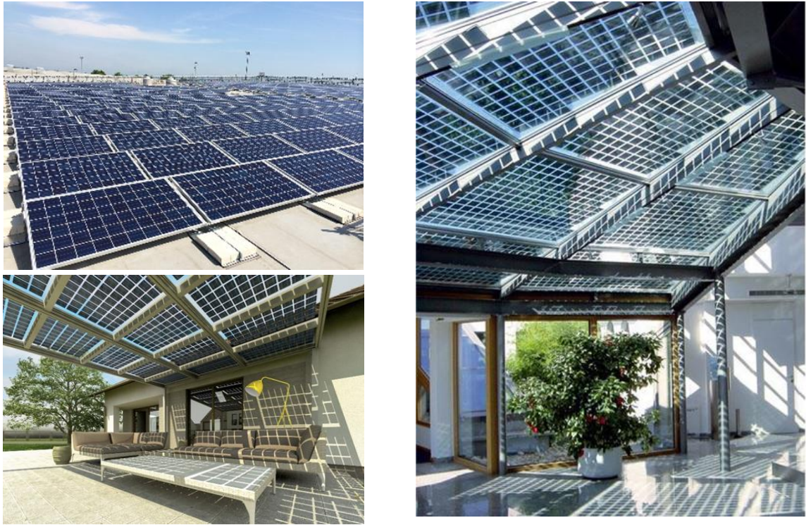
Figure 6 – Examples of PV installations
